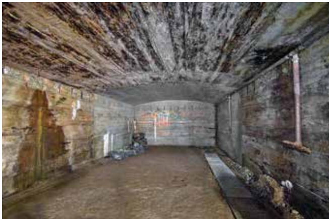
Roughly completed side chamber at Włodarz. The comparatively poor standard of finish implies the huge speed at which the project was being advanced.
